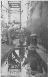
On the docks the wharfingers boosted turnaround efficiency by improved handling methods. Whenever possible the hoses were lined up ahead of time; the tankers could load shortly after docking.
